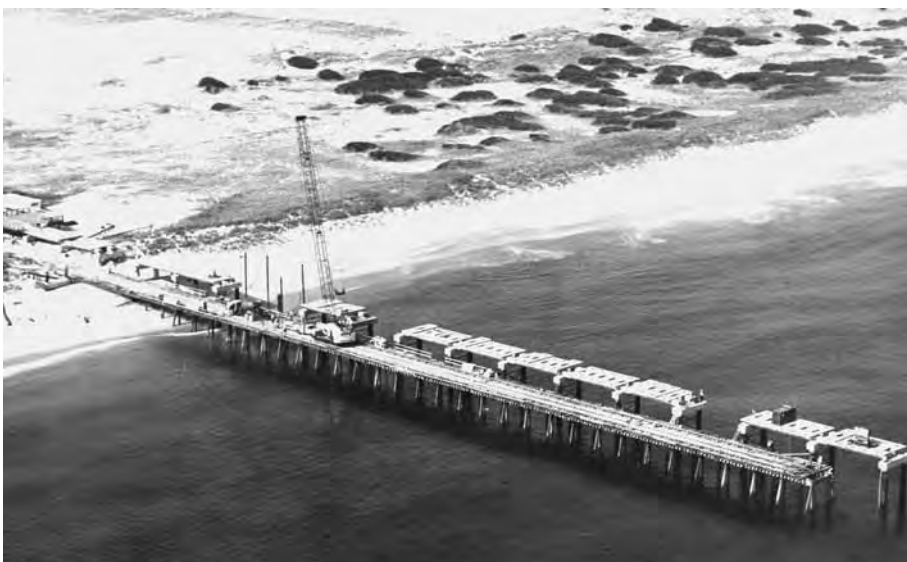
Construction of "the Pier" in the late 1970s at the Field Research Facility, located near Duck on the Outer Banks, N.C. The facility was part of the Coastal Engineering Research Center, established in 1963 to study coastal engineering problems. After several moves and reorganizations, the center became part of the Coastal and Hydraulics Laboratory of the Engineer Research and Development Center.
