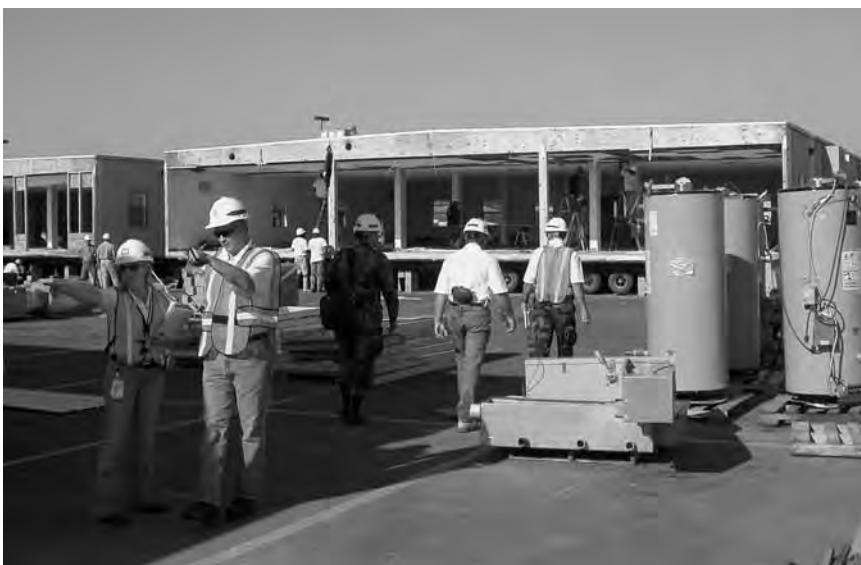
Corps of Engineers personnel supervising the placement of a community health facility in Chalmette, La., October 2005.
