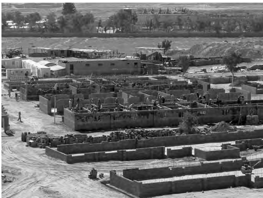
Barracks take shape at the Afghan army's Central Corps headquarters at Pol-e-Charki. Building the army facilities was the first major construction program in Afghanistan in decades, August 2003.
