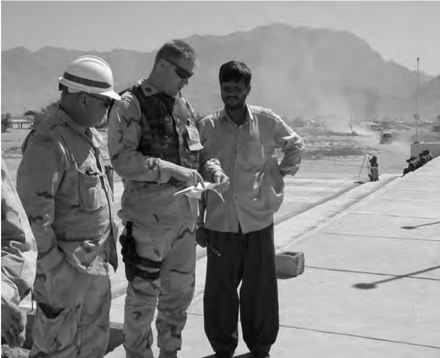
Cpt. Chris Beck of the Afghan Area Office discusses the construction of the Afghan National Army facilities at Pol-e-Charki, August 2003.
