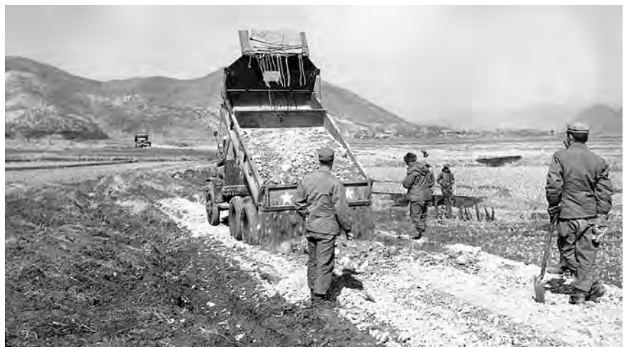
Men of the 65th Combat Engineer Battalion reinforce a muddy road on the north bank of the Han River, March 1951
