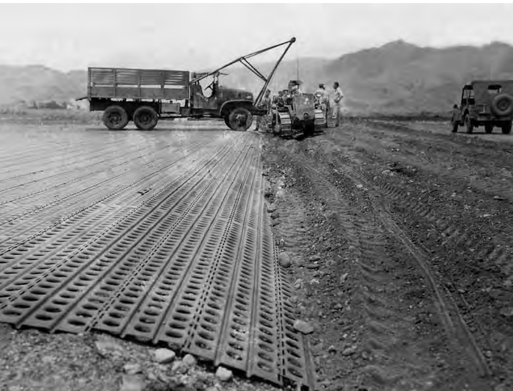
Engineers lay pierced-steel plank to construct a runway rapidly in New Guinea, February 1944
