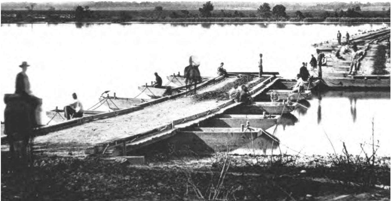
Ponton bridge under construction at Aiken's Landing on the James River, summer, 1864.
