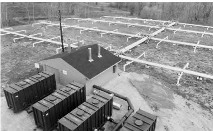
The volatilization system that removed dangerous organic compounds that contaminated ground water around the Twin Cities Ammunition Plant, Minn.
