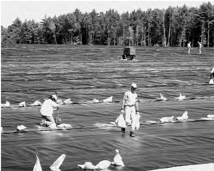
Geo membrane and gas vent layers covering a landfill at K. I. Sawyer Air Force Base, Mich., 1996
