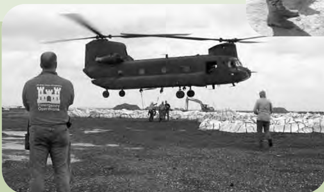
Chinook helicopter prepares to lift 5,000-pound sandbags to repair damaged flood walls.
