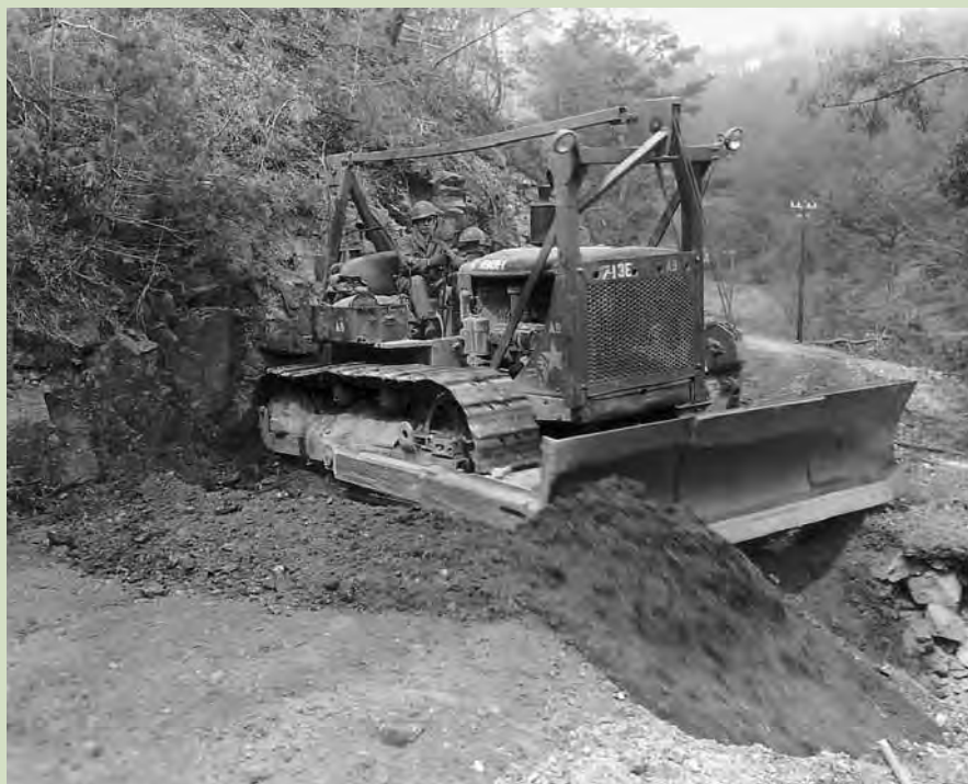
An engineer uses a bulldozer to repair a road damaged by retreating enemy troops. National Archives
