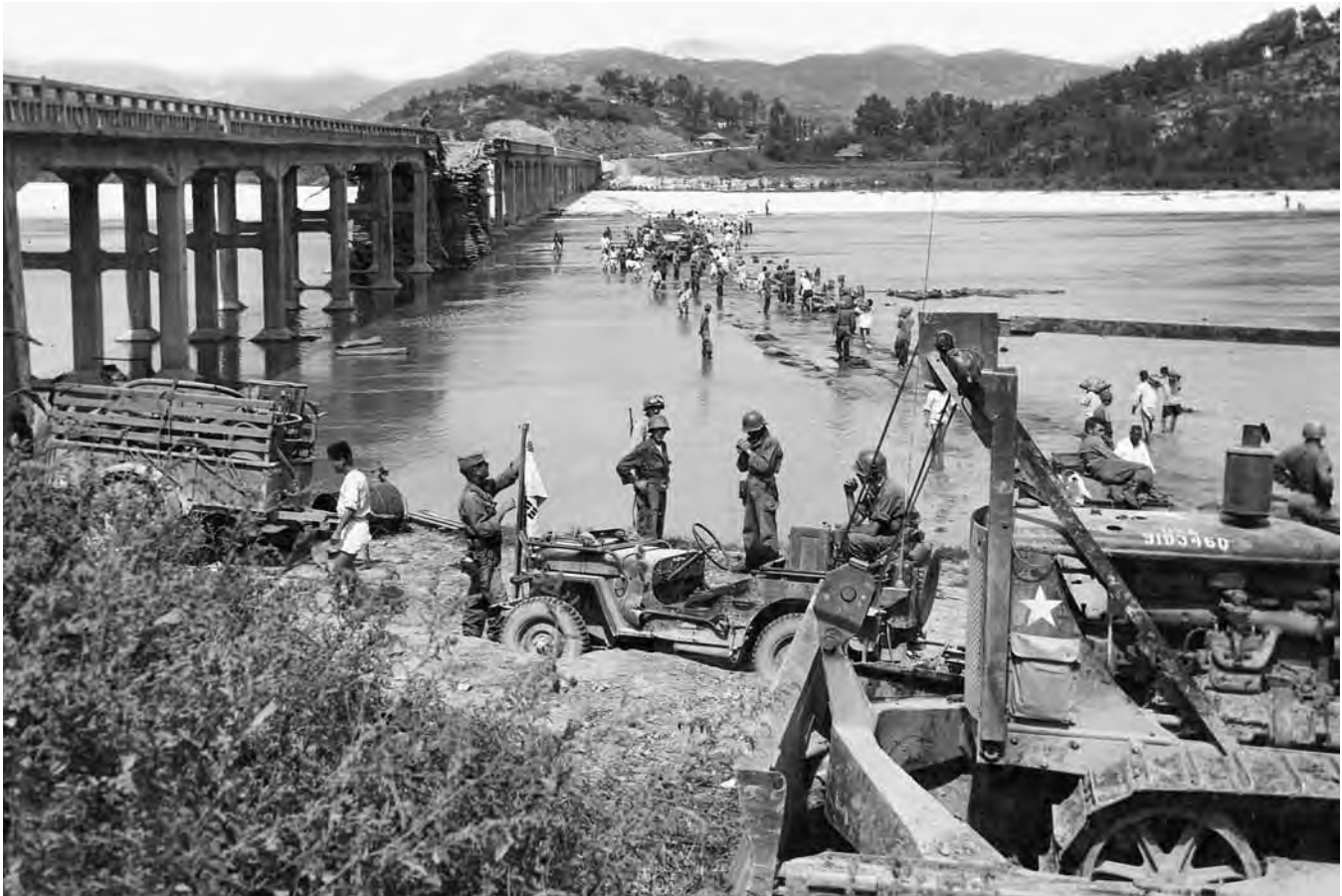
Engineers of the 2d Infantry Division construct a bypass to enable heavy equipment to cross the Hwang-gang River, 25 September 1950
