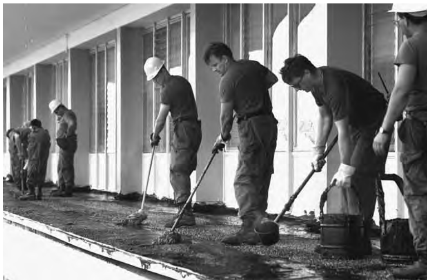
Military personnel repair the roof of a school damaged by Hurricane Andrew's strong winds.
