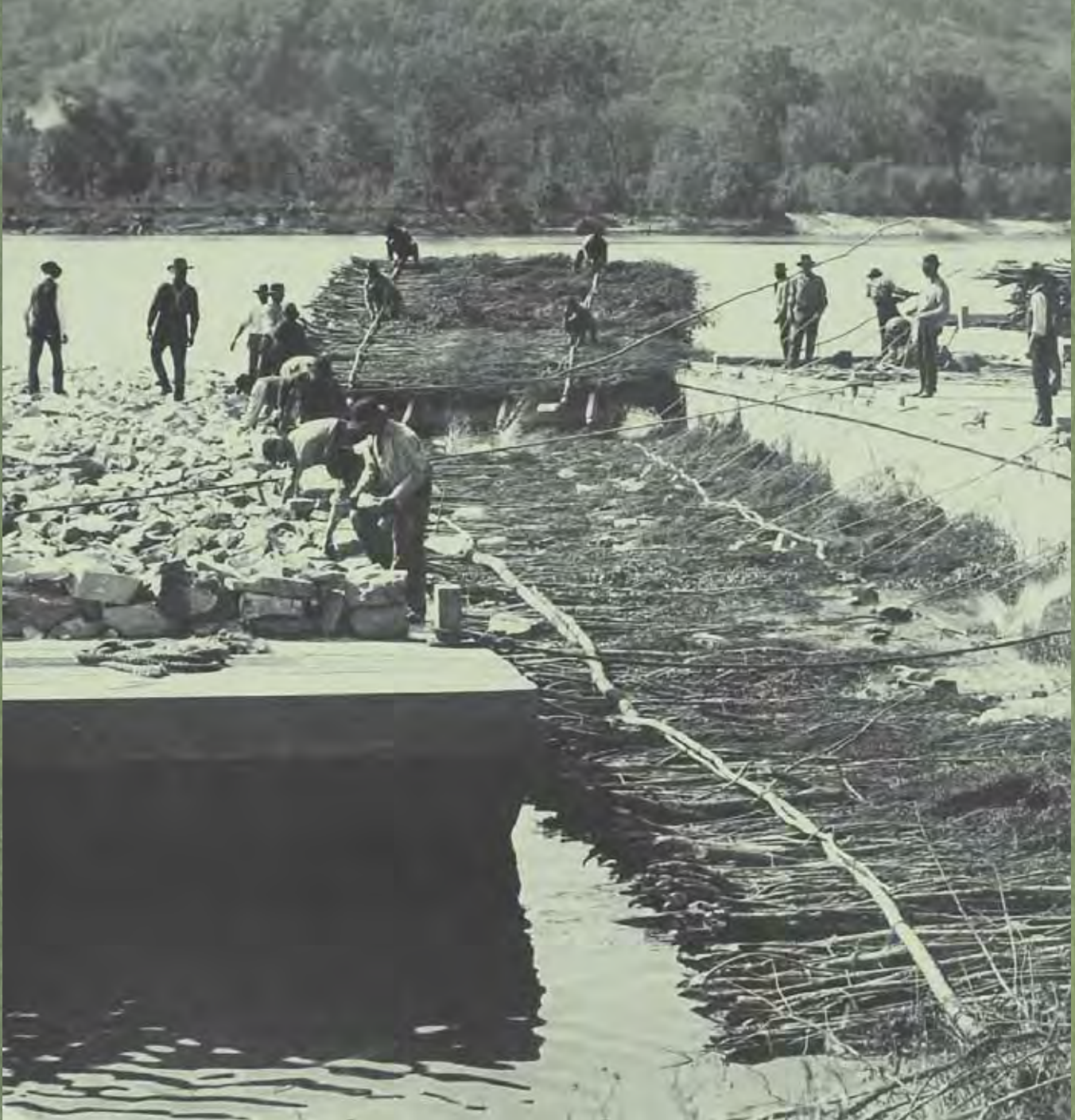
Construction of rock and brush wing dams on the Mississippi River in 1891. The photographer, Henry Peter Bosse (1844–1903), worked as a civilian engineer and draughtsman for the Corps of Engineers during the reshaping of the Mississippi River for modern transportation. Rediscovered only in the early 1990s, Bosse's photographs have won international acclaim, earning him a place among the J. Paul Getty Museum's "38 Photographers of Genius."
