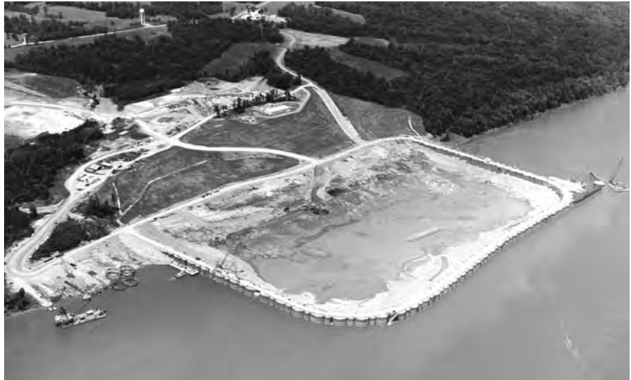
Completion of the dewatering of the cofferdam at the Olmstead Locks and Dam in Illinois, which took forty days, August 8, 1995
