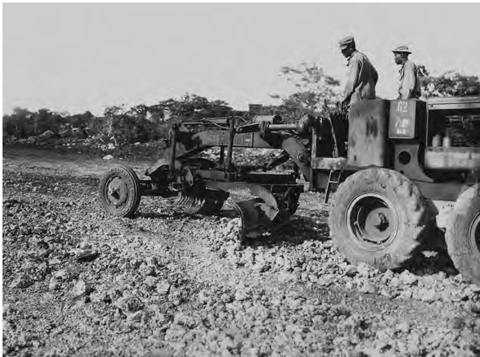
Engineers of the 856th Engineer Aviation Battalion, an African-American unit, grading an airfield on Kiriwina Island, east of New Guinea, October 1943.
