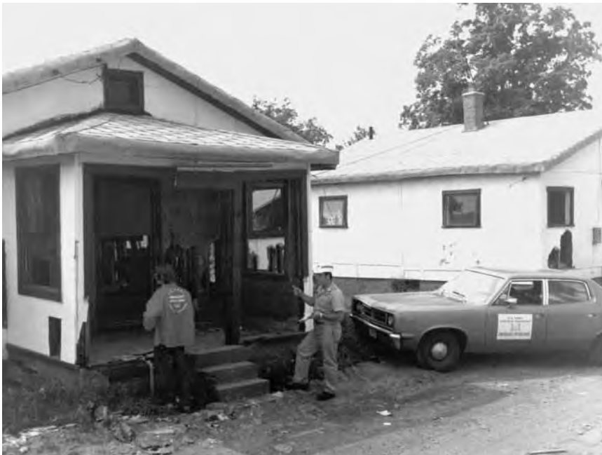
A Corps of Engineers disaster survey team inspects damaged homes following Tropical Storm Agnes.
