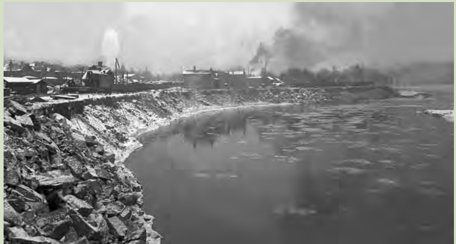
(above) View of eroded bank below abutment, Allegheny River, Dam 3, Jan. 1907
